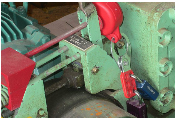
Switches and lockouts
